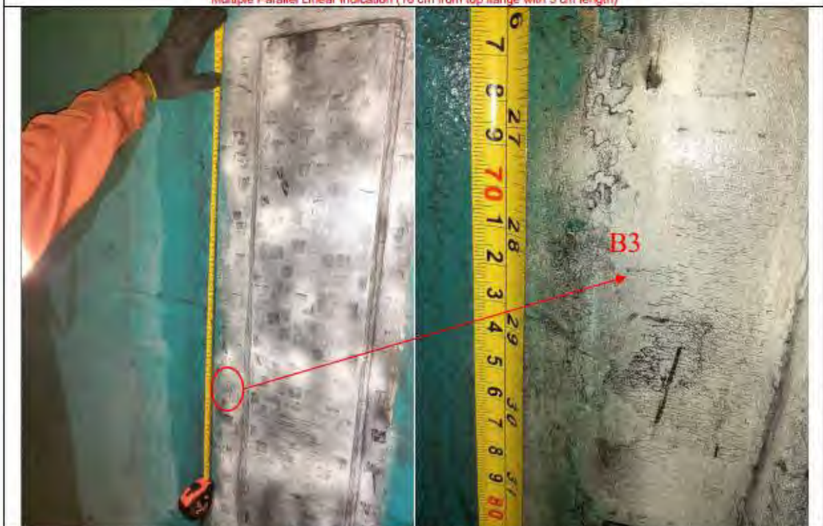
FIGURE 6: Item B – Web / B3 Indication Multiple Parallel Linear Indication (70 cm from top flange with 9 cm length)
